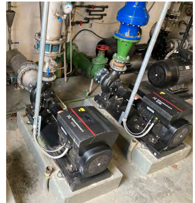
Replacement of water supply pumps with high efficiency pumps at our Lindau, Germany facility
